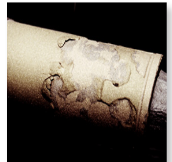
Failed Coating due to undercorrosion
